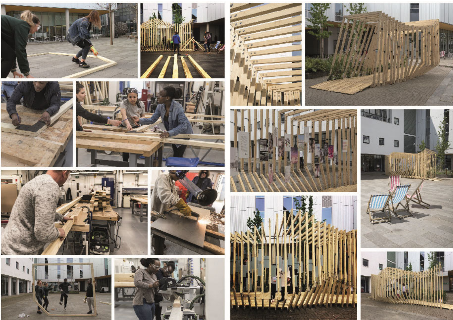
Figure 7. The Edge Pavilion workshop and final installation. Photo credit: Roger Forman, Guido Robazza.
