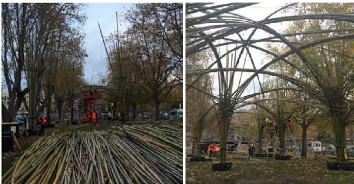
Figure 3: Central bay of canopy (left) and column and beam junction (right). Images: Helen Norrie.
